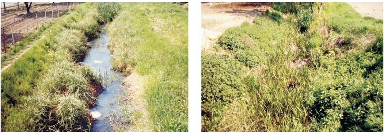
Picture 10. State of the drainage channels
